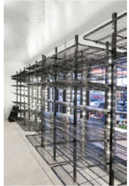
Standard Shelving Installed
